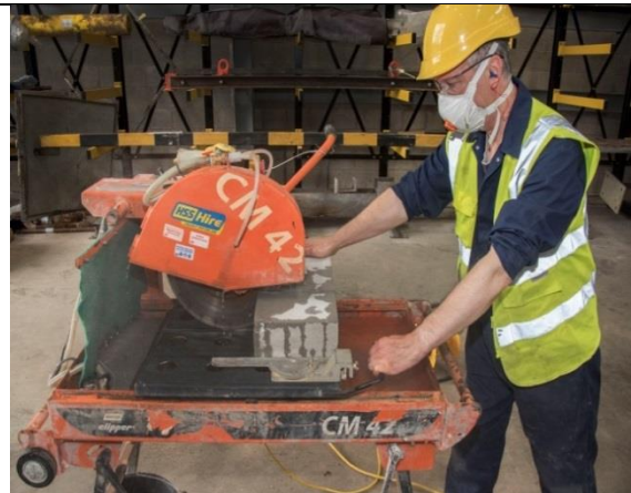
Good practice – Use of water suppression (shown) and RPE worn by the operator (HSE, GB)
