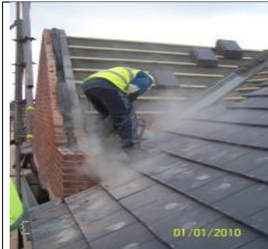
Poor Practice – Cutting roof tiles without control measures (National Federation of Roofing Contractors Ltd, GB)
