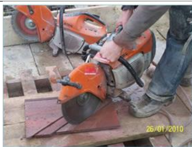
Good practice – Cutting roofing tiles with a tile cutter (National Federation of Roofing Contractors Ltd, GB)
