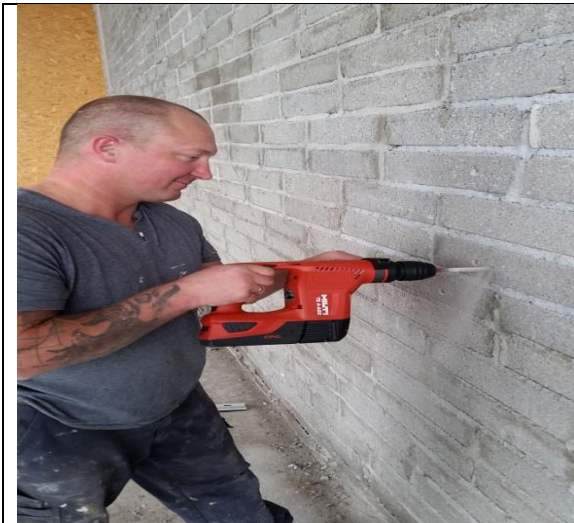
Poor practice – Using Hand-held drill with no on-tool extraction (David Flynn Ltd, IE)
