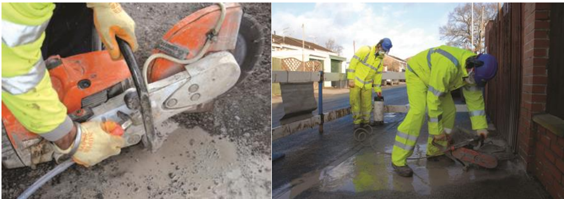
Figure 2 photographs showing water suppression system: (source HSE, GB)
