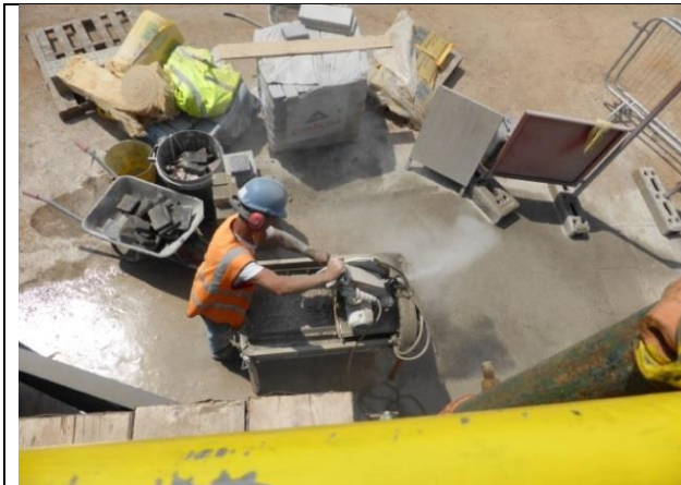
Poor Practice – No/insufficient water suppression and lack of RPE (HSE, GB)
