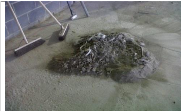
Poor Practice – Removal of rubble using dry sweeping (HSE, GB)
