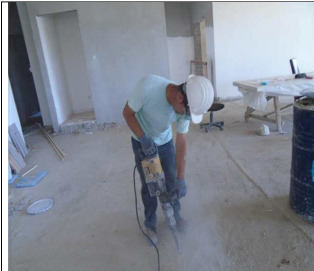
Poor Practice – Using a hand-held breaker without on-tool extraction (DLI, CY)
