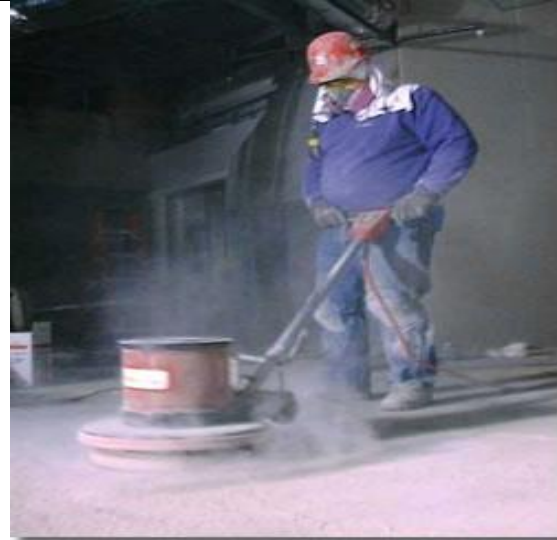
Poor Practice – sanding concrete floors without on-tool extraction (GDWW, B)
